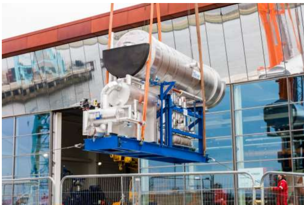
Figure 10 – A river source heat pump (2,600 kW heating capacity) delivered to Queens Quay, Clydebank
