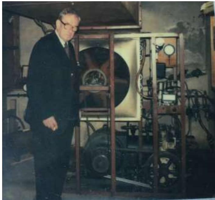
Figure 5 – Dr JW Macfarlane and his heat pump in the basement of Cartbank
