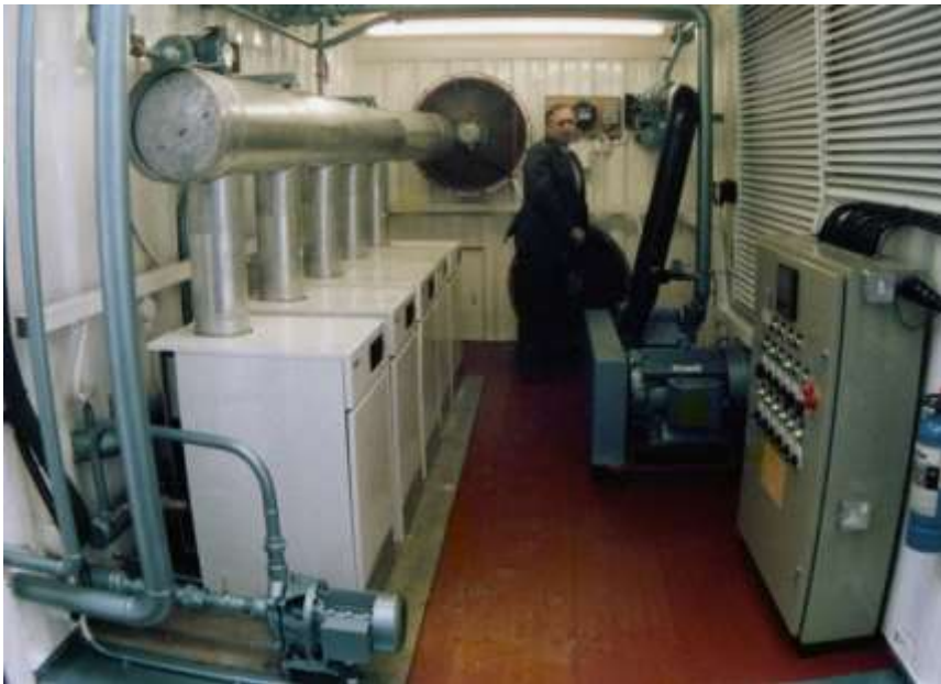
Figure 8 – Dr SF Pearson’s factory heat pump with 5 gas boilers and R22 compressor on the right
